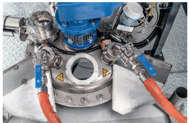
Reactor prepared for cleaning mode: the spray lances are plugged in.
